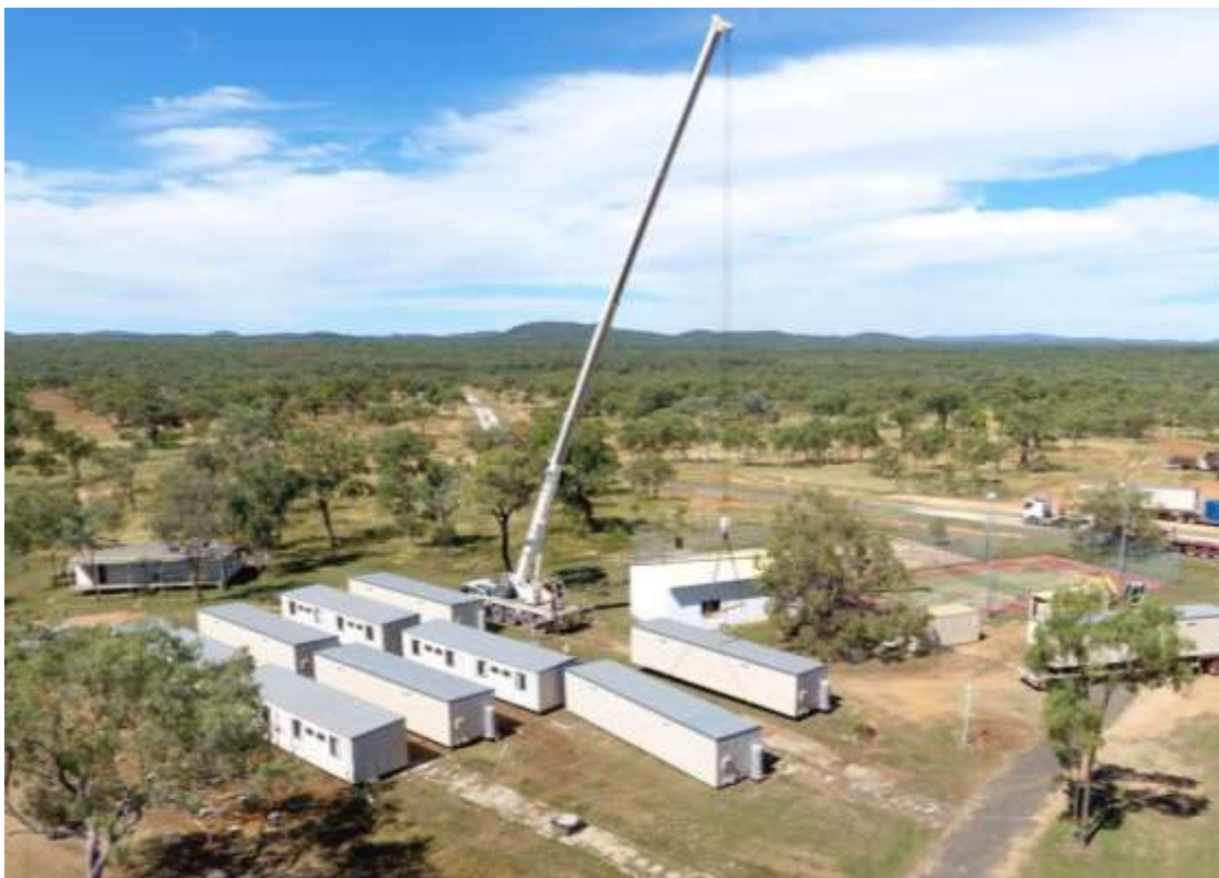
Figure 1: Expansion of accommodation camp at Oaks Rush, Kidston
